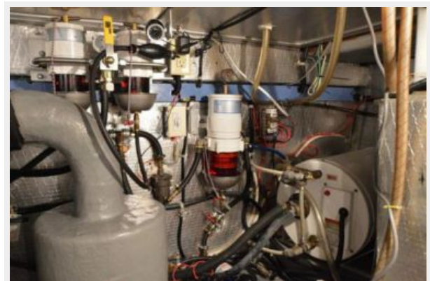
Fuel Scrub System
