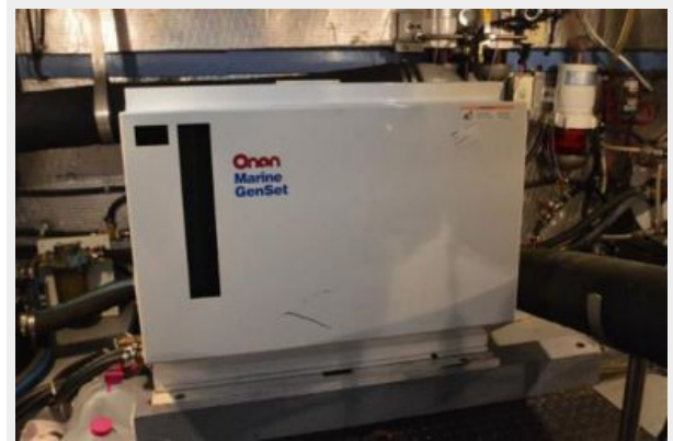
Generator in Sound Shield
