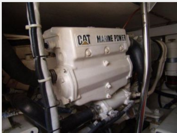
Engine & Mechanical Equipment 3
