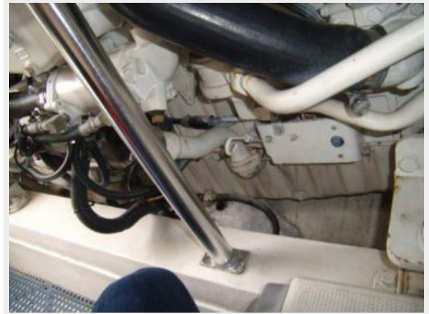
Engine & Mechanical Equipment 2
