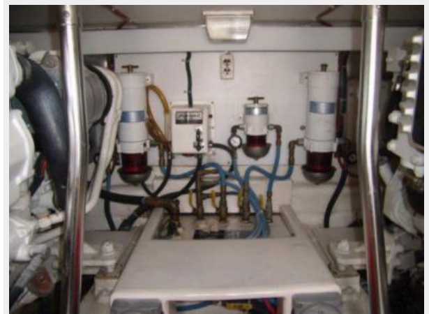
Engine & Mechanical Equipment 4
