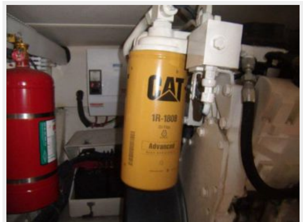
Engine & Mechanical Equipment 6
