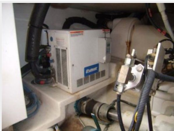
Engine & Mechanical Equipment 5
