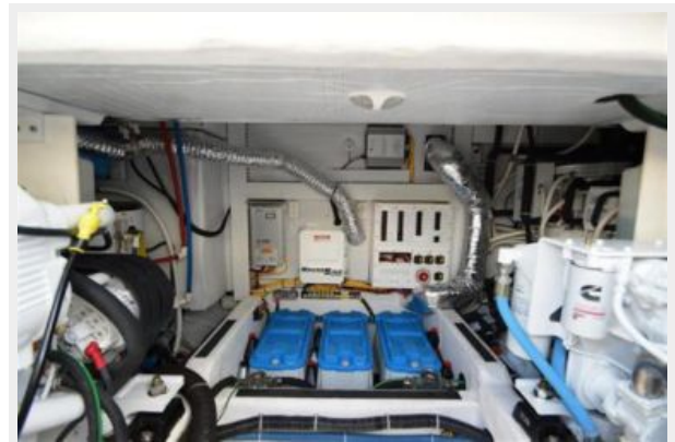
Engine Room Electrical
