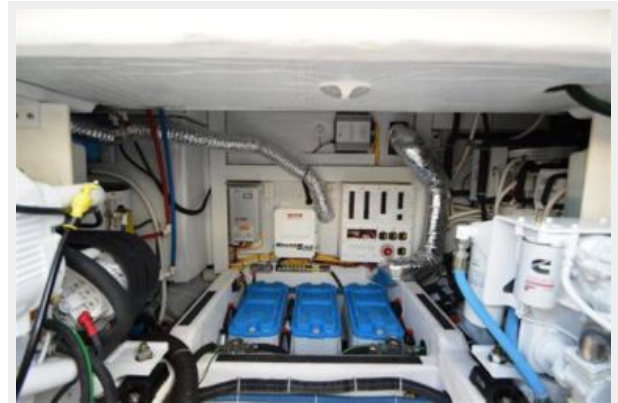
Engine Room Electrical
