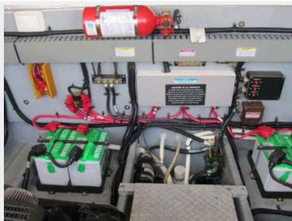
33' Sea Ray engine room forward
