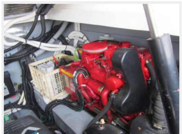
33' Sea Ray generator
