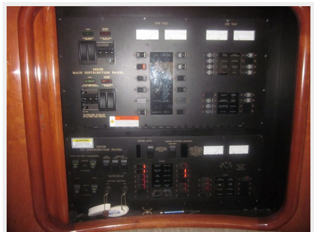
Salon Electrical Panel
