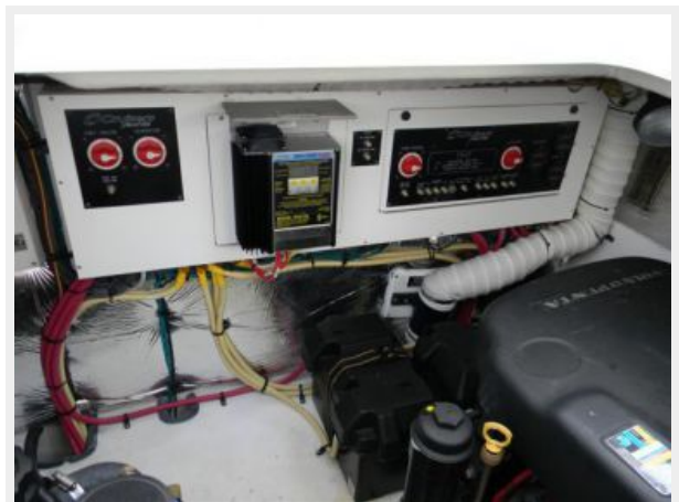
Engine Room Electrical
