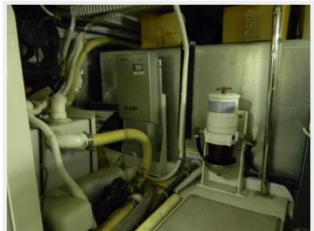
Engine Room Equipment
