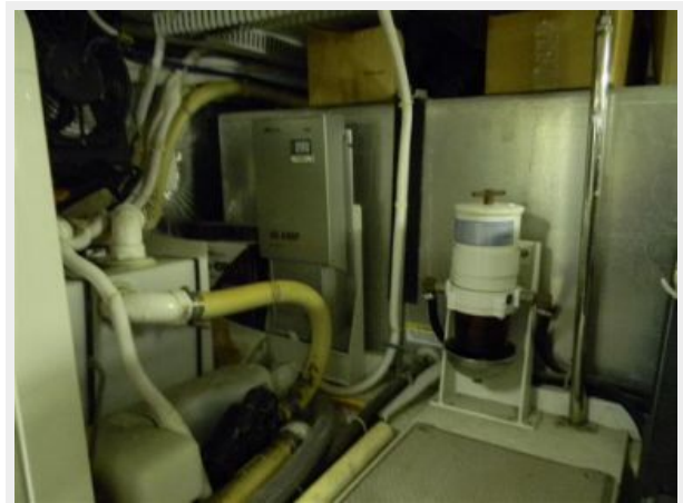
Engine Room Equipment
