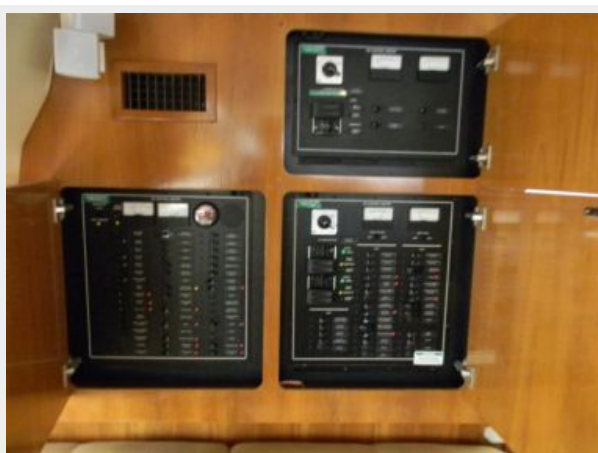
Electrical Distribution Panel
