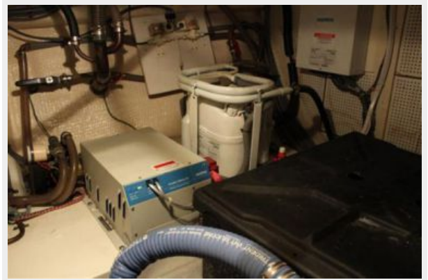
Clean Mechanical Space
