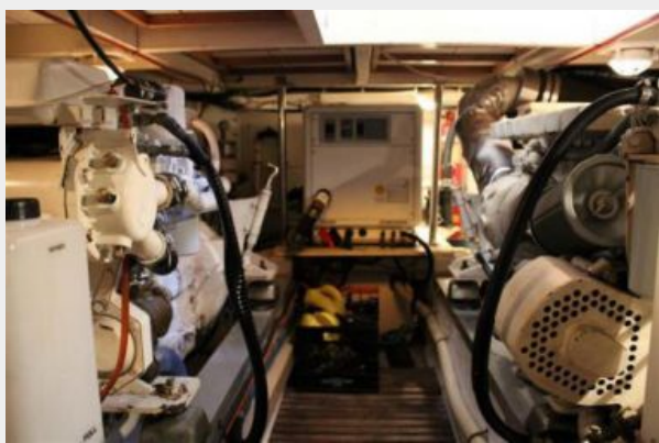
Engine Room Looking Aft
