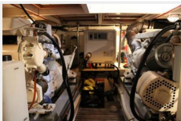
Engine Room Looking Aft
