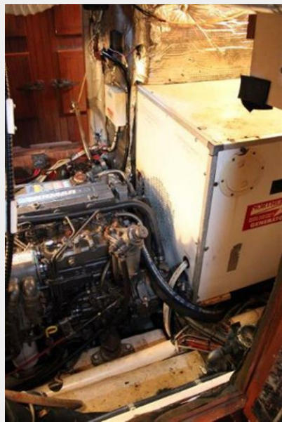
8kw Northern Lights Generator
