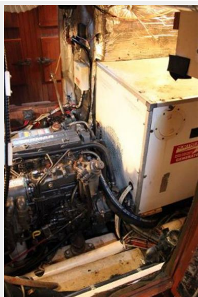
8kw Northern Lights Generator
