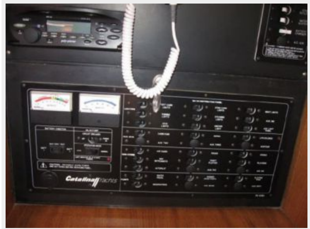
Electrical Panel at Nav Area
