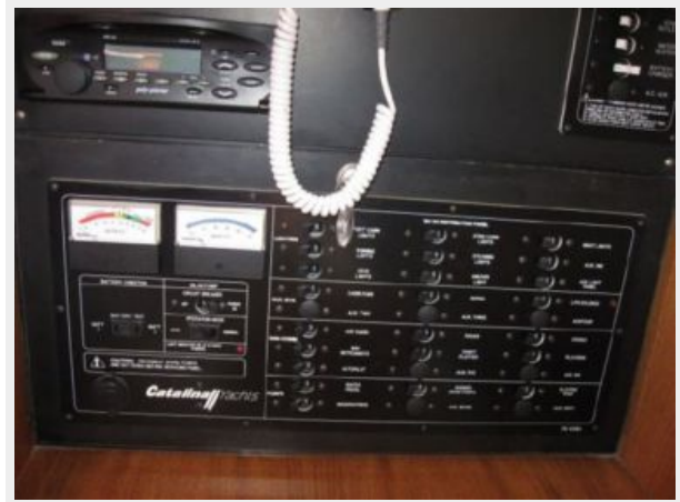
Electrical Panel at Nav Area
