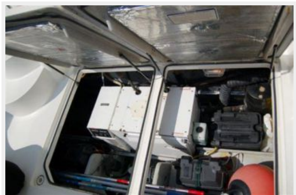
Cockpit-Genset and Storage
