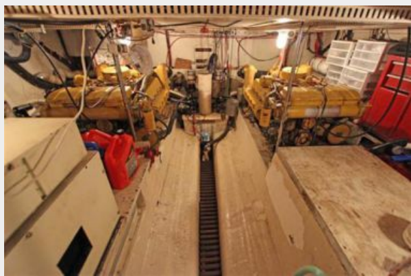
Engine Room Looking Aft
