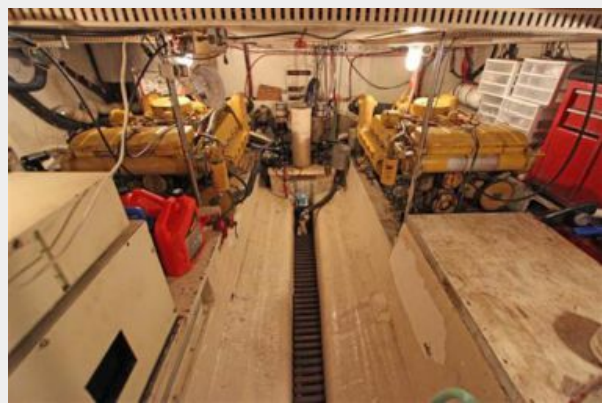
Engine Room Looking Aft
