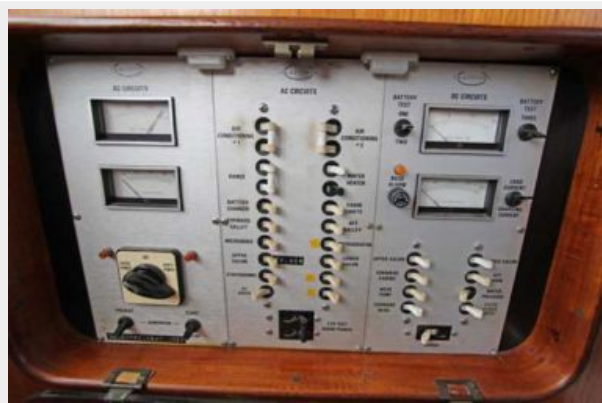
AC/DC Electrical Panel
