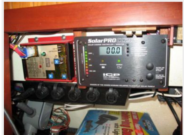
Solar panel controls and charger
