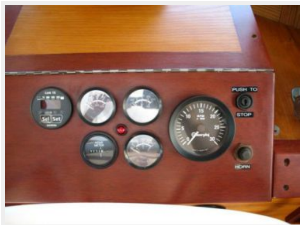
Main engine panel
