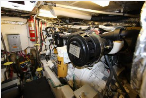
Engine Room Starboard Forward
