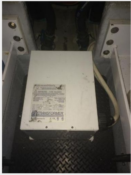
Engine Room - Facing Aft
