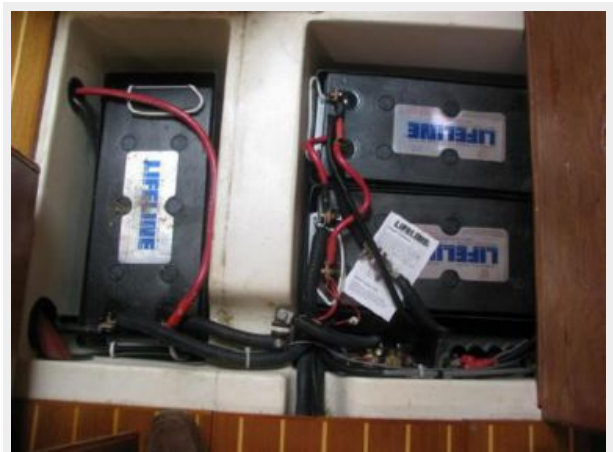
3 of 5 AGM 4D house batteries
