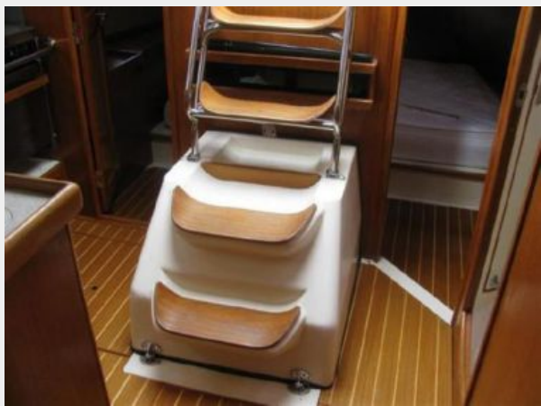
Engine access under companionway steps.
