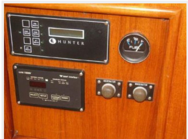
Batteries and Tank level monitors
