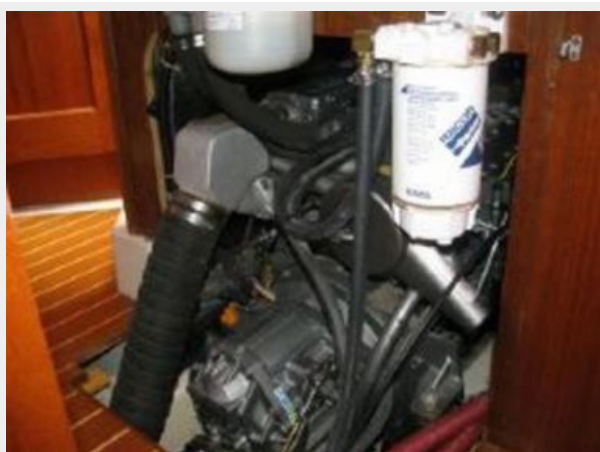
Back of engine access from master cabin
