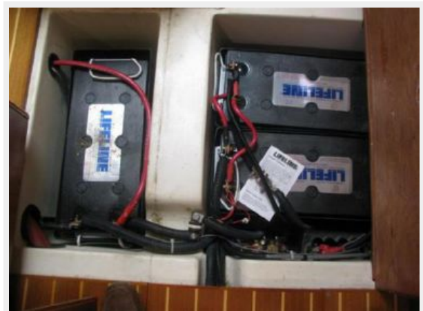
3 of 5 AGM 4D house batteries
