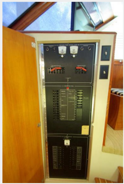
Power Distribution Panel
