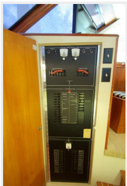
Power Distribution Panel
