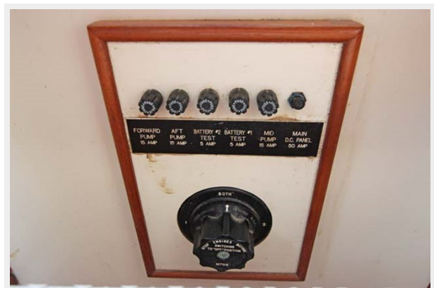
Battery Switch & Fuse Panel
