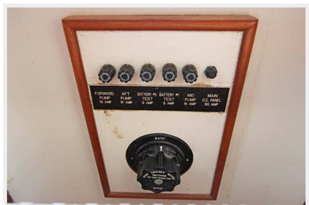
Battery Switch & Fuse Panel
