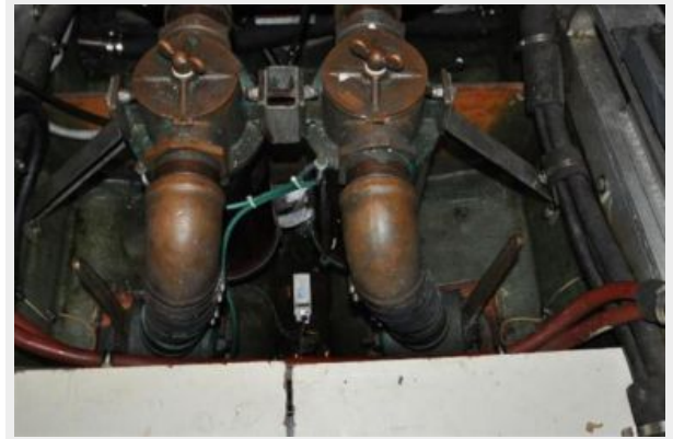
main engine intakes
