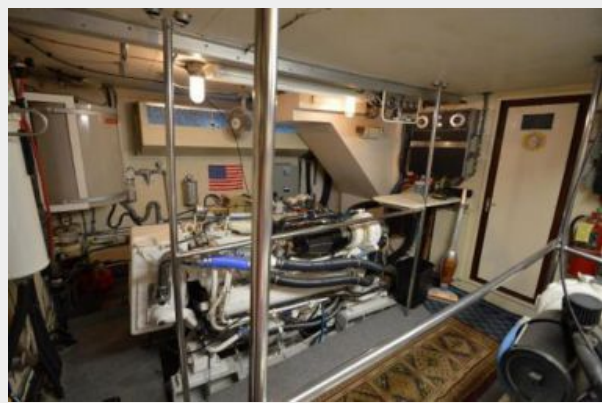
Engine Room Starboard
