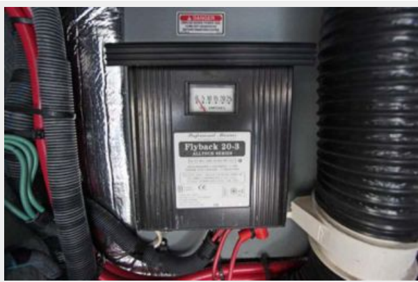
20 Amp Marine Battery Charger
