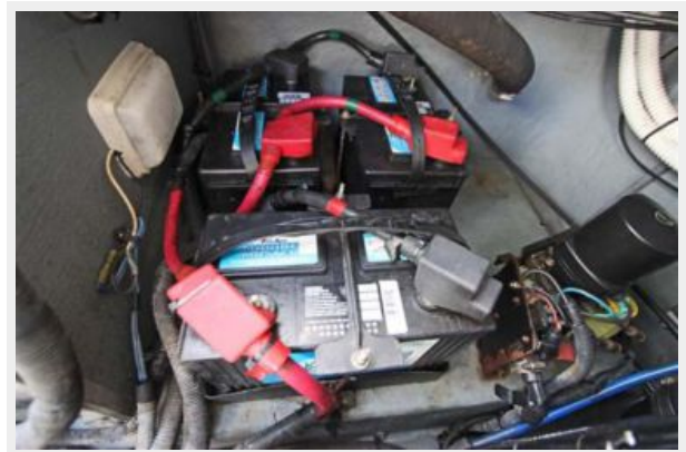
3-Group 24 Marine Batteries
