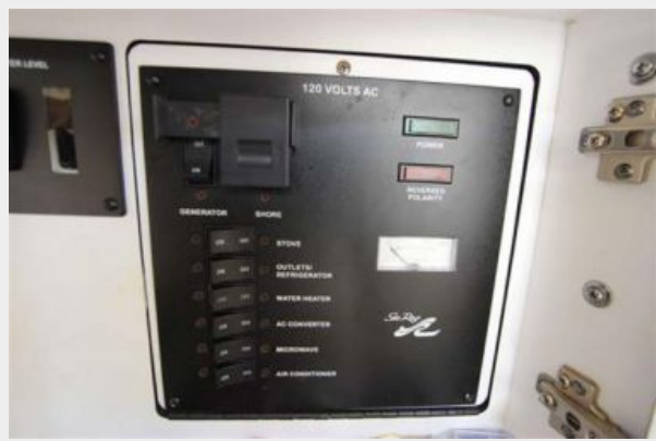
AC Electrical Panel
