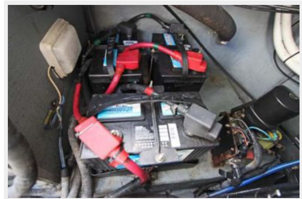
3-Group 24 Marine Batteries
