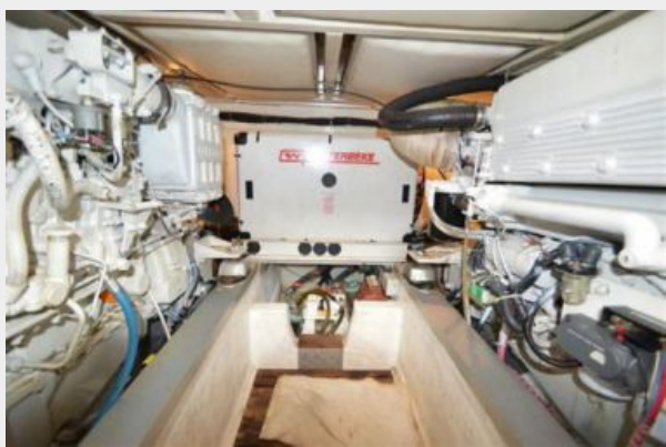
Engine Room Aft
