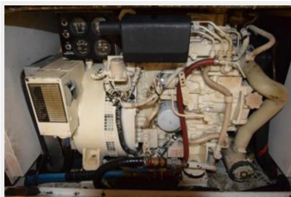
Generator w/o Sound Shield
