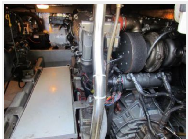
Engine Room Starboard
