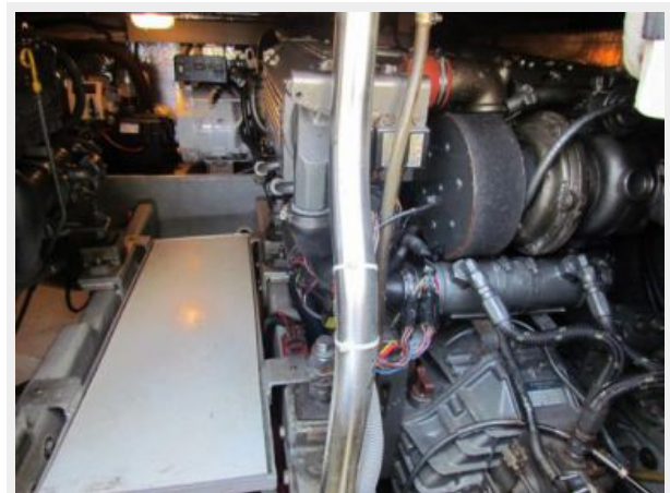
Engine Room Starboard
