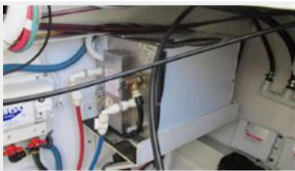
Hot Water Heater
