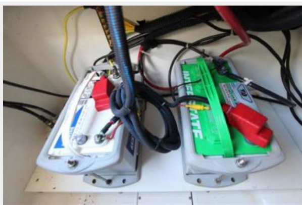
Dual Batteries Mounted In Center Console
