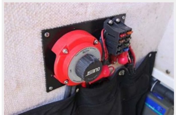
Guest Battery Switch
