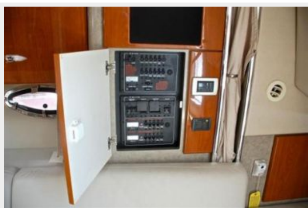
Main Electric Panel
