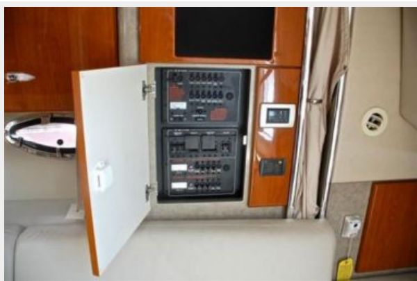
Main Electric Panel
