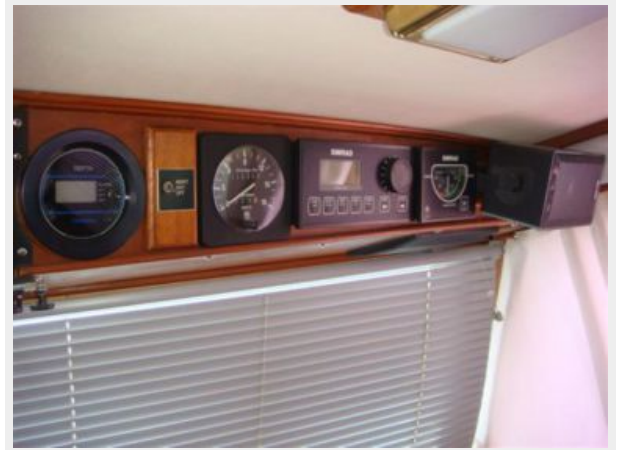
44' DeFever lower helm overhead electronics photo1
