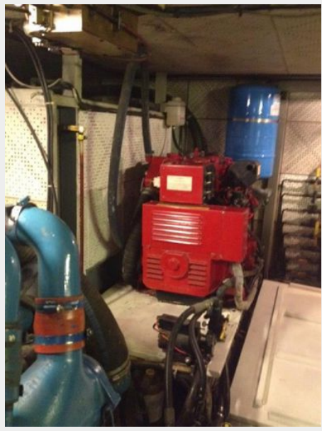
44' DeFever engine room starboard aft
