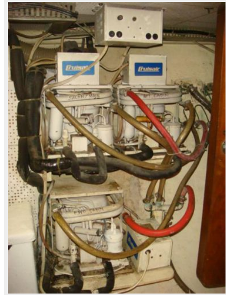
44' DeFever air conditioning system
