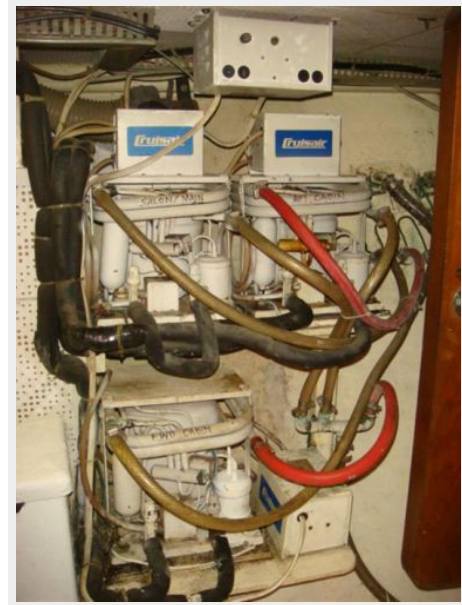
44' DeFever air conditioning system
