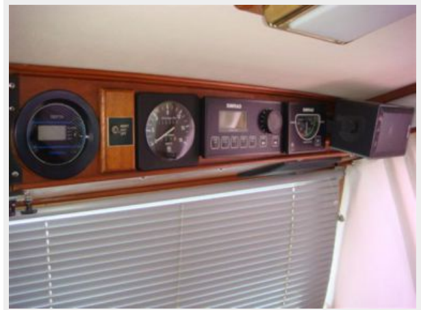
44' DeFever lower helm overhead electronics photo1
