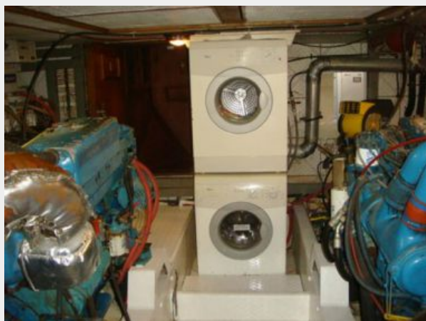
44' DeFever engine room forward
