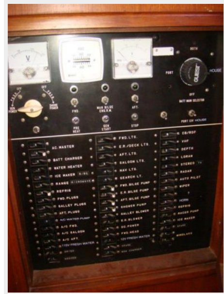
44' DeFever electrical panel
