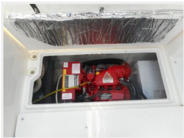
28' Bayliner generator access
