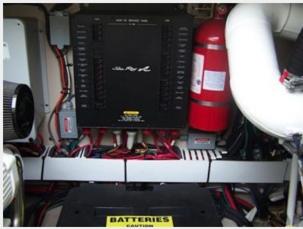
Engine Room Equipment
