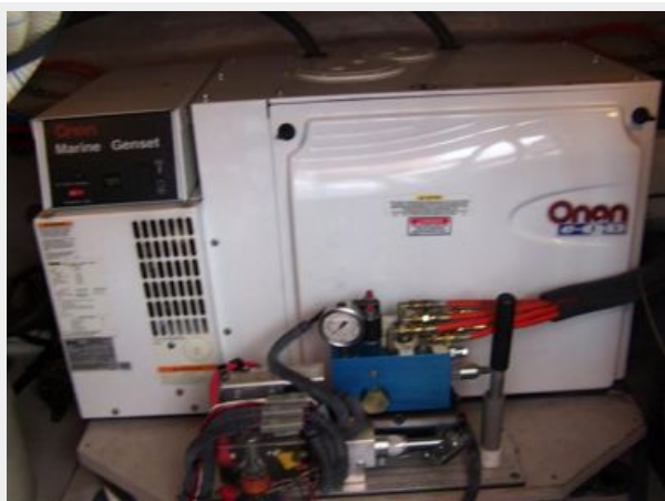
Generator w/ Sound Shield
