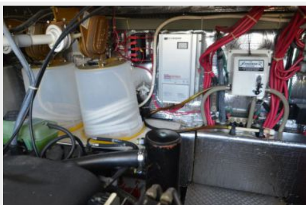
'03 Regal 3860; Cable masters, Battery Charger, & Oil Change System
