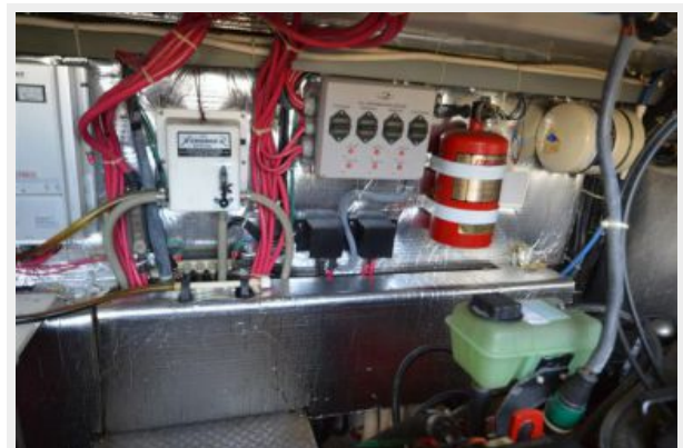
'03 Regal 3860; Fire Suppression System
