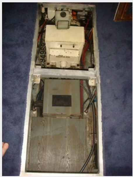
38' Carver engine room access
