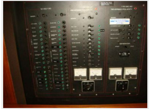
38' Carver electrical panel
