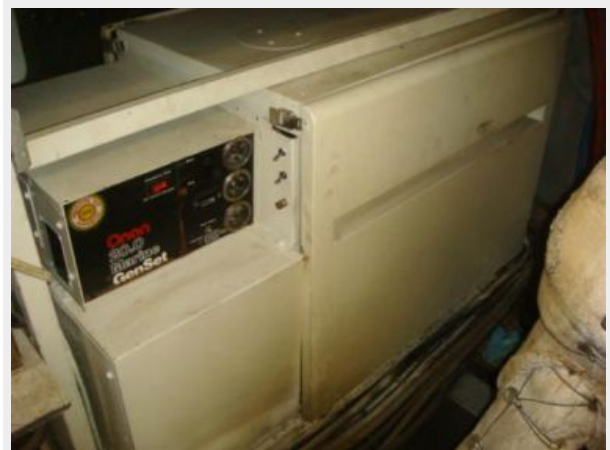
55' Cheoy Lee port generator
