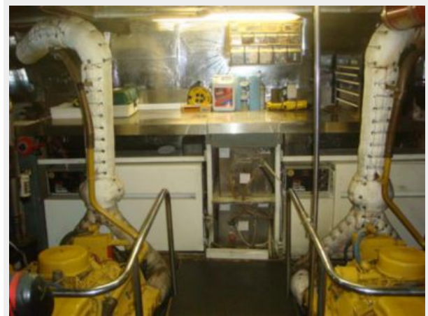
55' Cheoy Lee engine room aft
