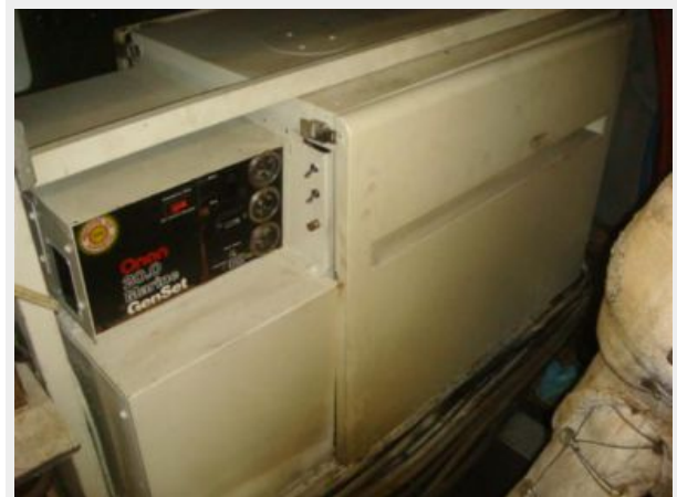
55' Cheoy Lee port generator
