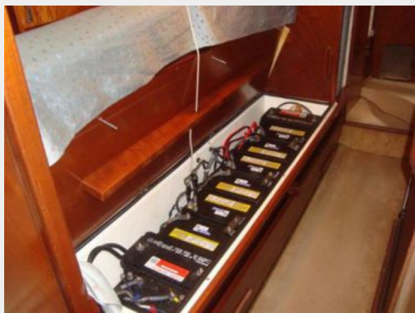
Battery Storage - Sea Berth
