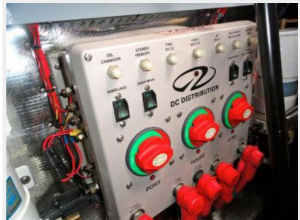
Engine Room Battery Bank
