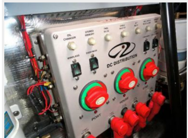
Engine Room Battery Bank
