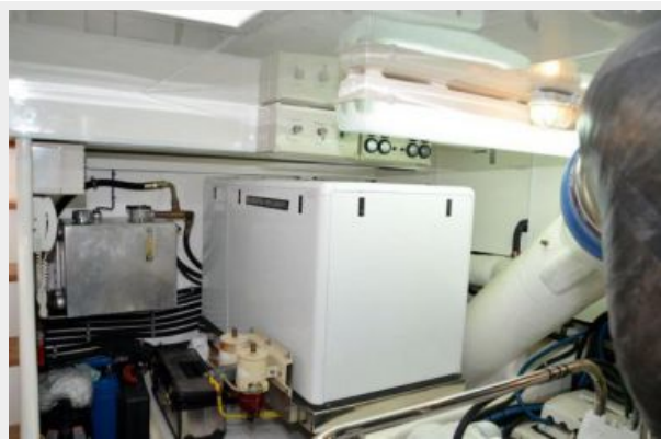
Engine Room Generator
